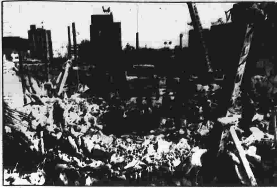
Work crews continue to clear rubble from the site of a building that collapsed April 23 in Bridgeport. The building's insurer has agreed to help pay for cleanup operations before liability for the collapse is determined.
